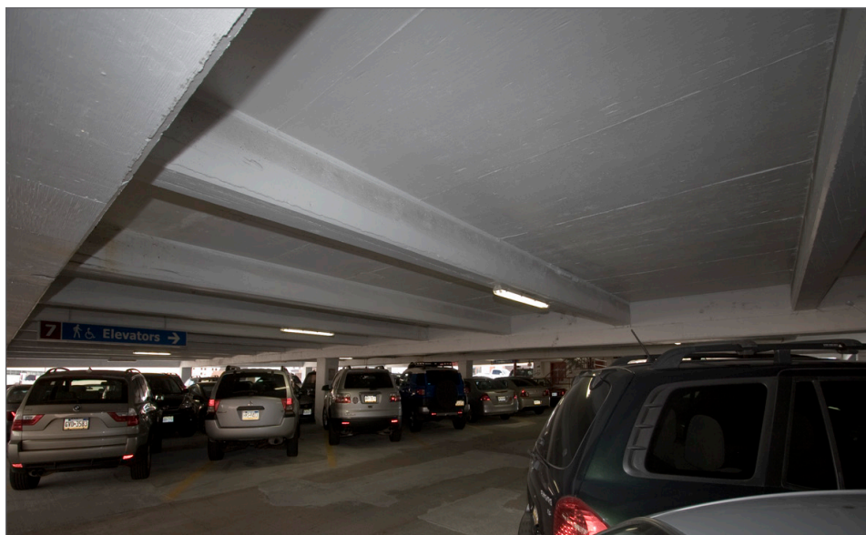
Miro reflector lighting system offers more light and better color rendering at the 12th & Walnut Streets Parkway Parking Garage
