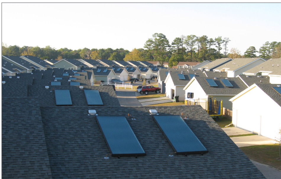
Solar water heating panels aboard the Marine Corps Base Camp Lejeune in Jacksonville, NC. FLS Energy photo
